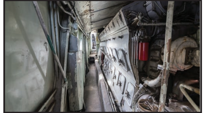
Inside of an engine room on a diesel train
