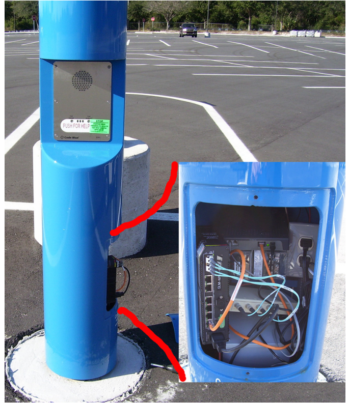
Magnum 6K Switch in typical Code Blue tower installation
